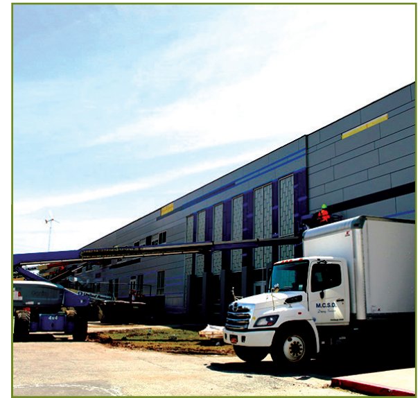
Construction is nearing completion on the steel frame exterior of the building.
